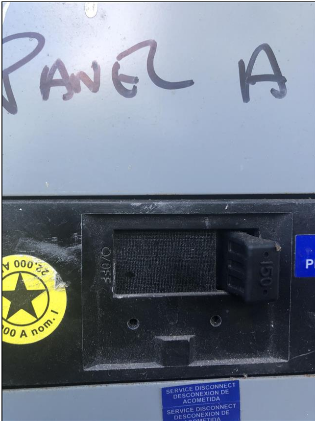
7.1 Item 1(Picture) 150 Amp Main Circuit Breaker
