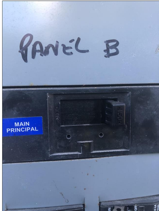
7.1 Item 2(Picture) 150 Amp Main Circuit Breaker
