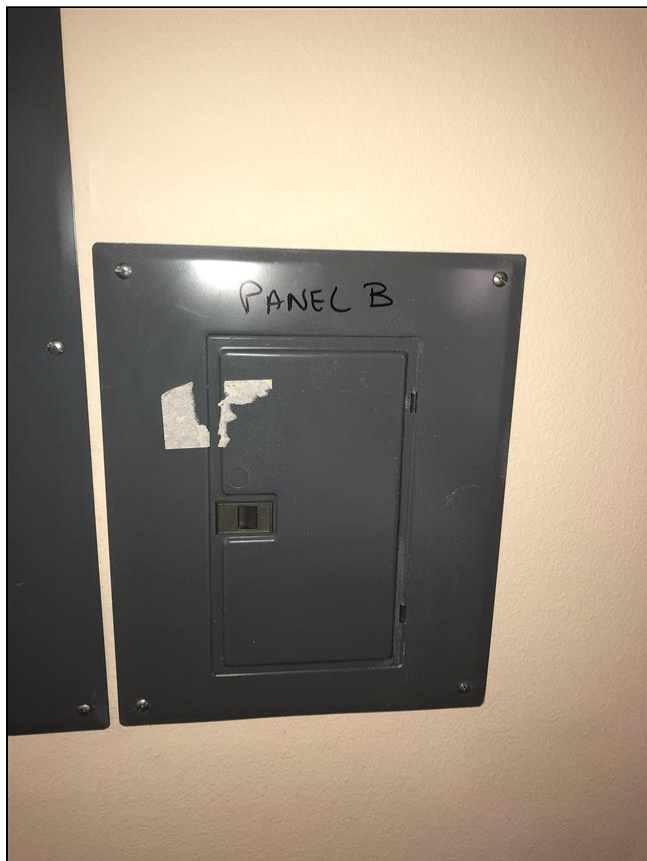
7.6 Item 7(Picture) Sub Electrical Panel B
