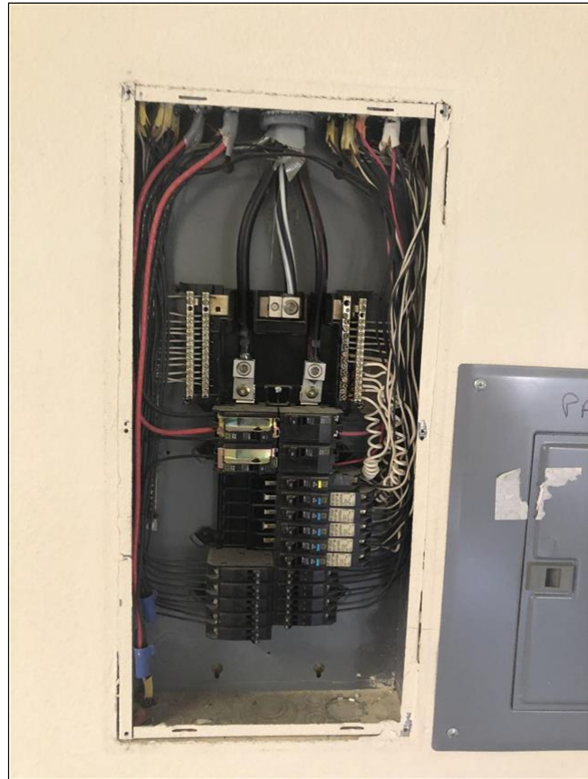
7.6 Item 6(Picture) Sub Electrical Panel A With Cover Removed
