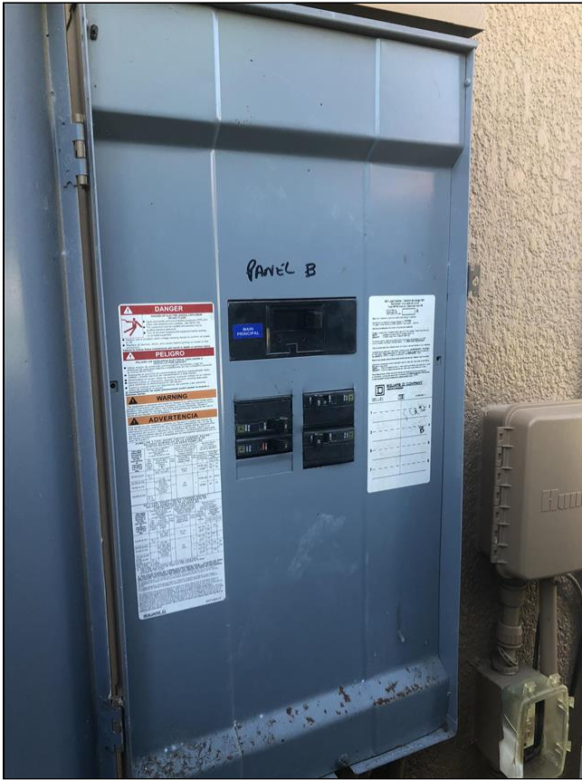
7.6 Item 3(Picture) Main Electrical Panel B
