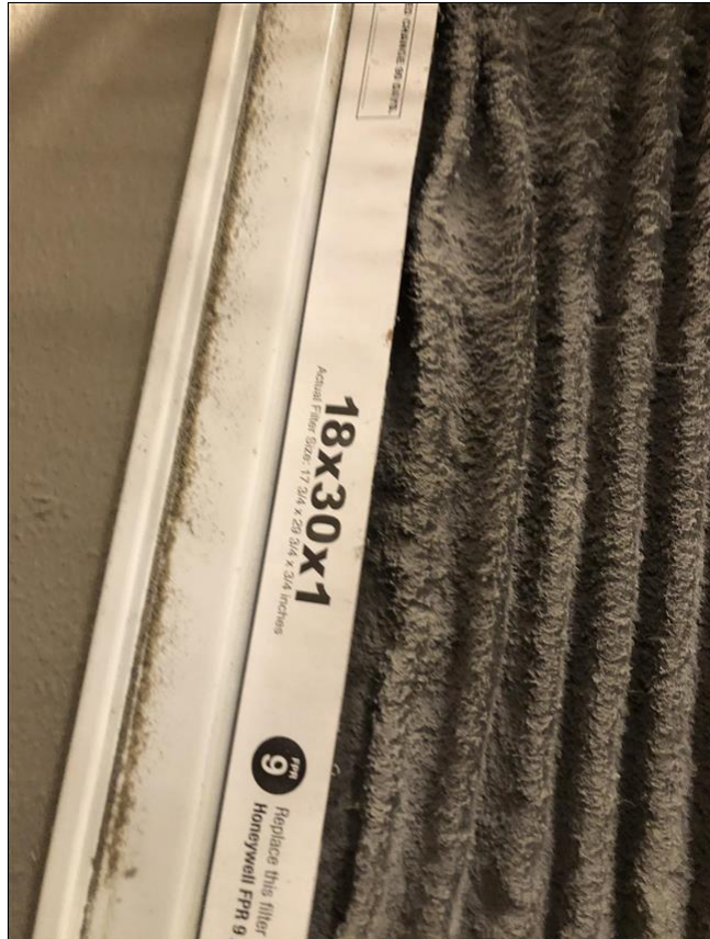
8.3 Item 2(Picture) Filter Dirty Needs Changed System #1
