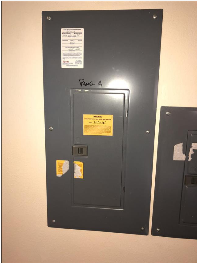
7.6 Item 5(Picture) Sub Electrical Panel A
