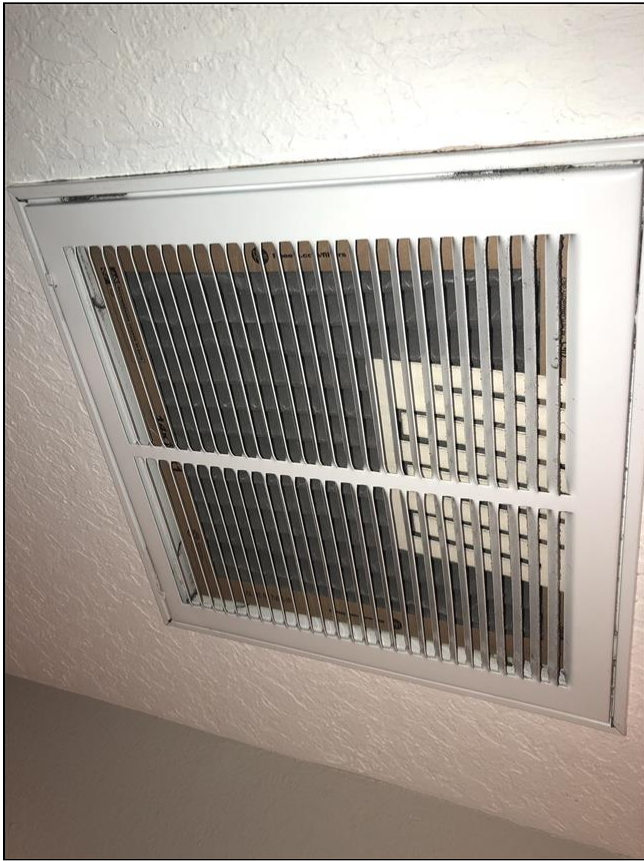
8.3 Item 3(Picture) System #2 Filter Location
