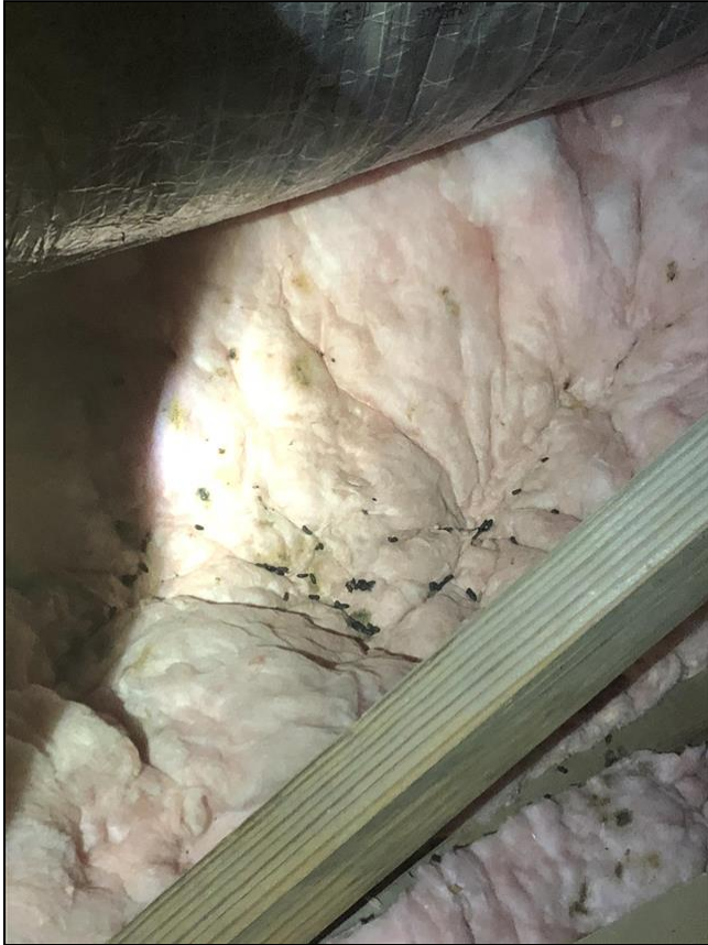
5.5 Item 1(Picture) Rodent Droppings
