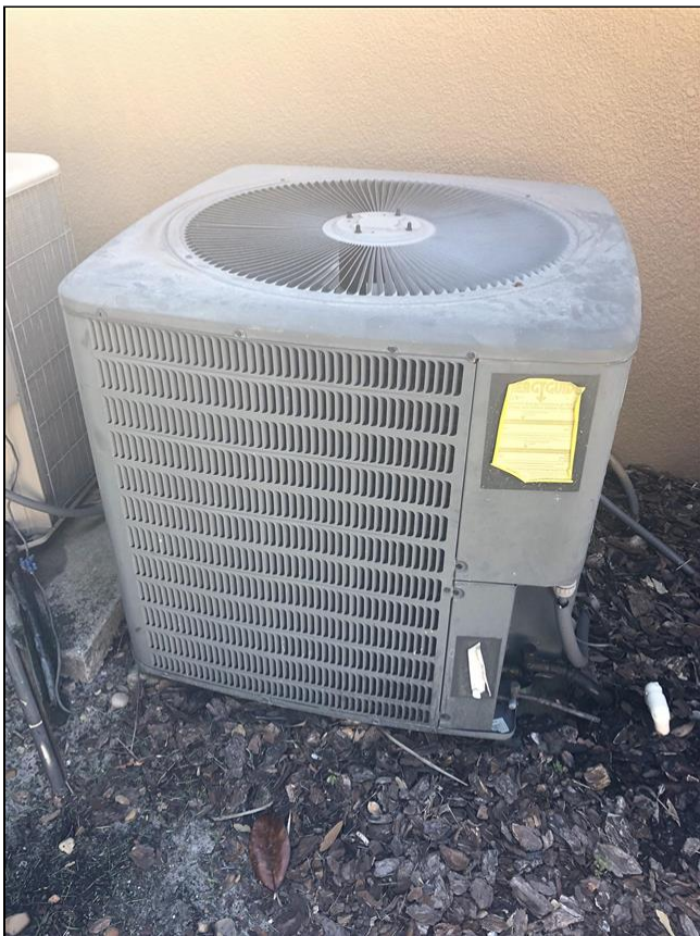
8.8 Item 1(Picture) Outdoor Heat Pump System #1
