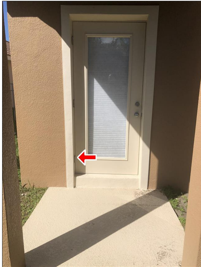
2.1 Item 4(Picture) Master Bedroom Exterior Door
