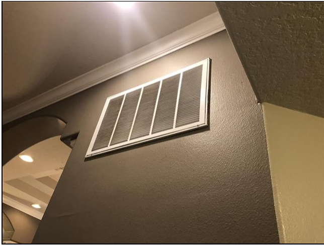
8.3 Item 1(Picture) System #1 Filter Location
