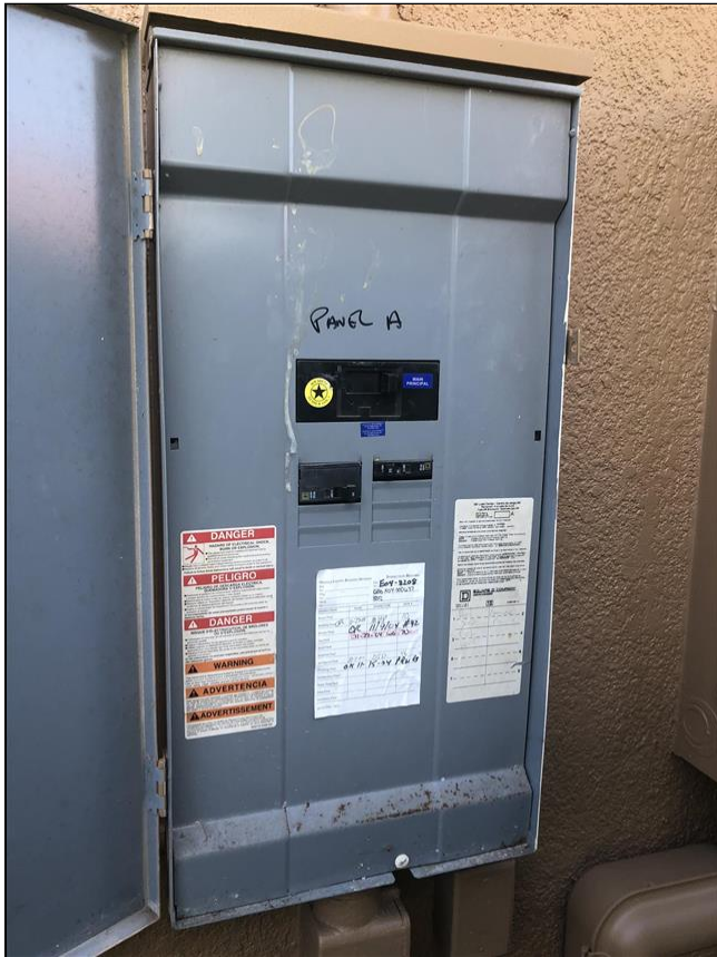
7.6 Item 1(Picture) Main Electrical Panel A
