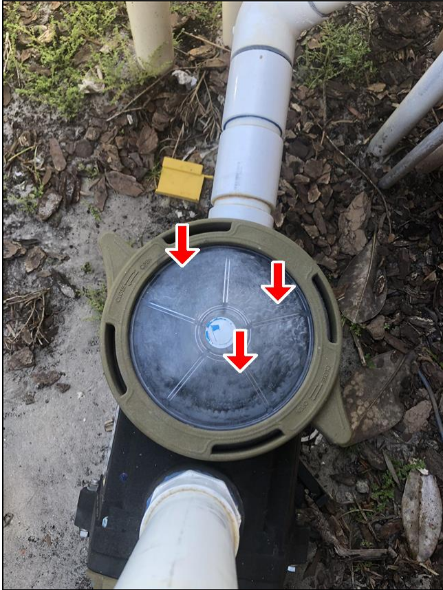
12.0 Item 1(Picture) Pool Pump
