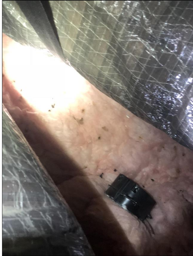
5.5 Item 2(Picture) Rodent Droppings
