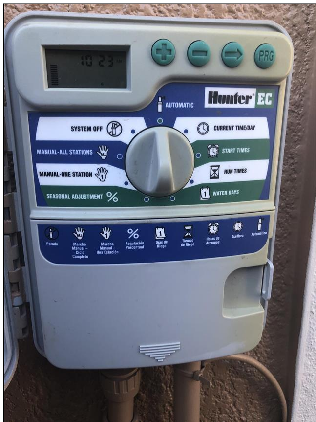
11.1 Item 1(Picture) Irrigation Controller North Side
