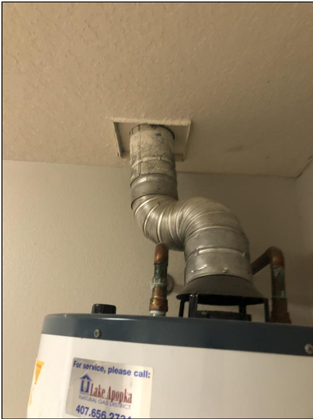
8.5 Item 1(Picture) WH Flue
