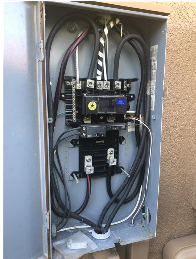
7.6 Item 2(Picture) Main Electrical Panel A With Cover Removed
