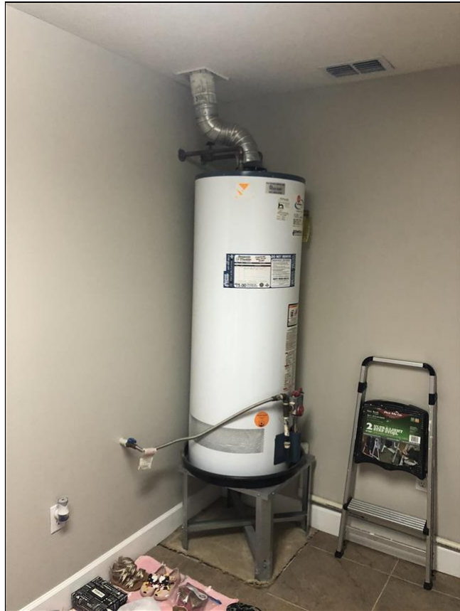
6.2 Item 2(Picture) Gas Water Heater
