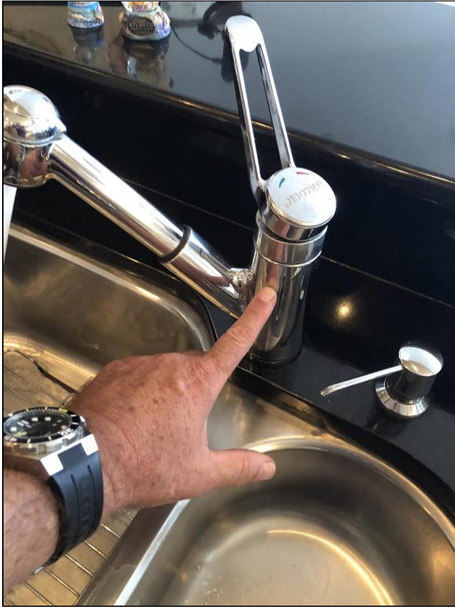
6.1 Item 2(Picture) Kitchen Sink Faucet
