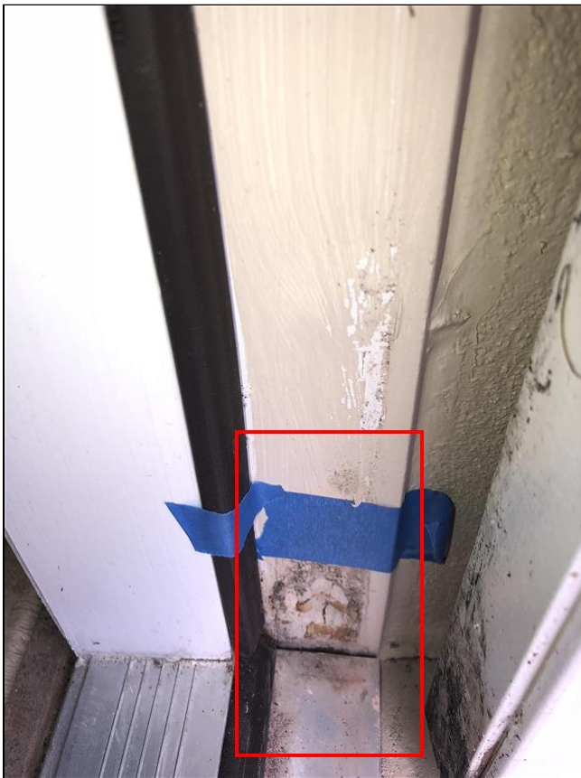
2.1 Item 1(Picture) Left Side Lower Frame Pool Bath Exterior Door
