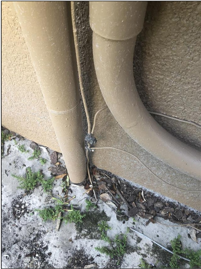
7.1 Item 3(Picture) Main Panel Ground Wire
